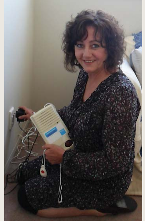
Carol installs a specially adapted security alarm into a high risk home.
